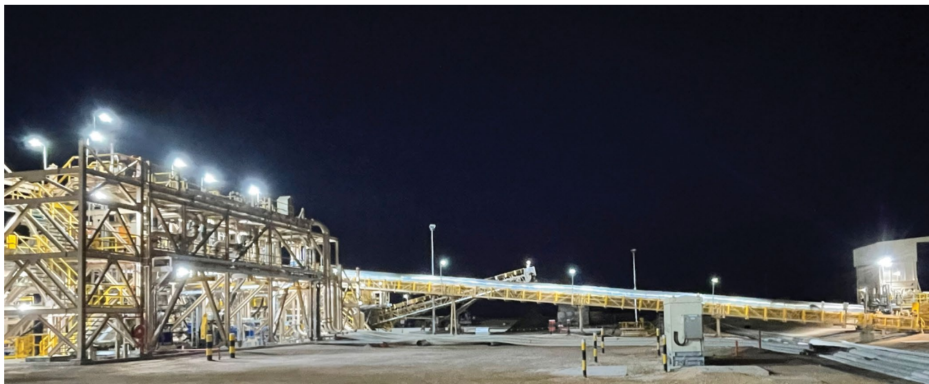
Mining has commenced at Balranald and heavy mineral concentrate has been produced.
