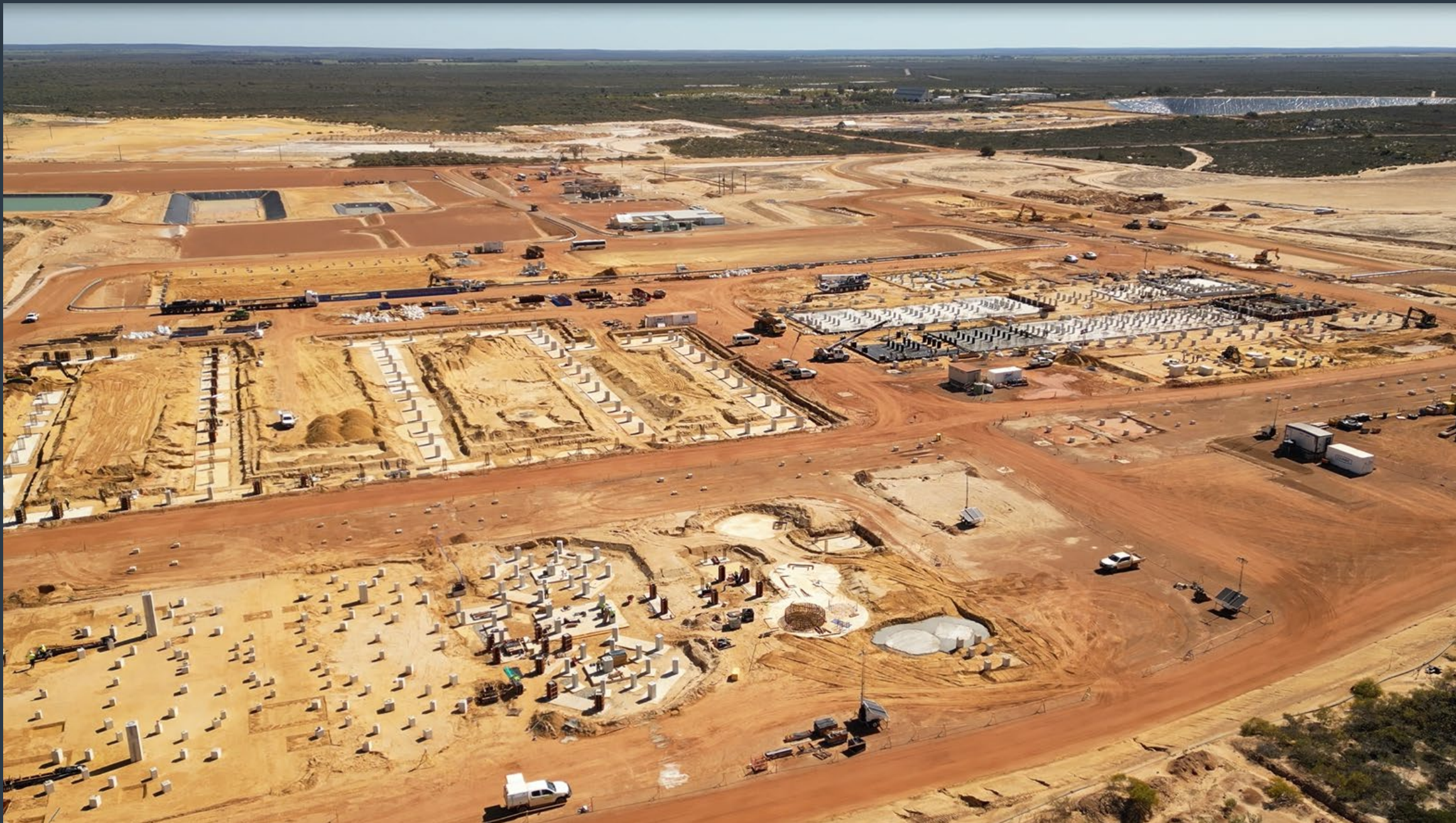
Eneabba rare earths refinery, Western Australia
