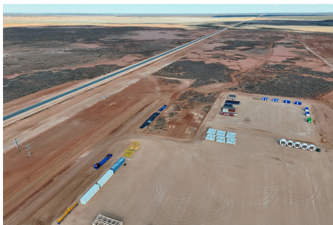
Aerial view of the sealed road with new deliveries in the mining panel area
