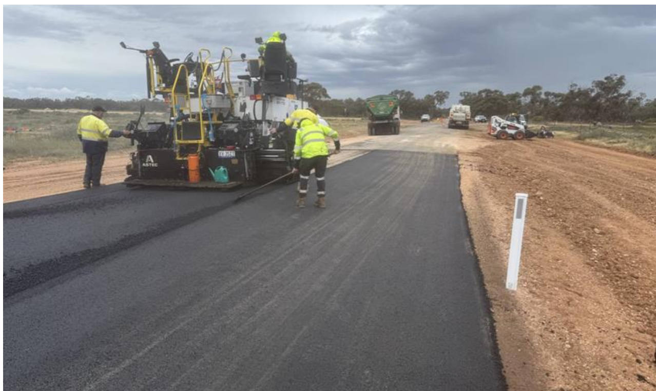
Photo 2: Public road upgrade and widening works of McCabe Street and Balranald-Ivanhoe Road intersection completed in September 2025.
